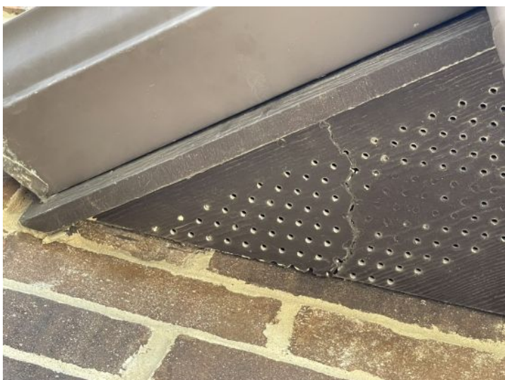
Cracked vent soffit. Monitor and repair if needed
