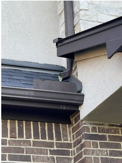
Downspouts discharging on roof covering. Recommend extending to discharge into first story gutters
