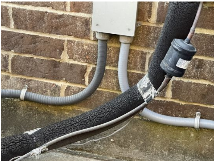
weather damaged insulation on HVAC return line. Replace insulation to maintain system efficiency.
