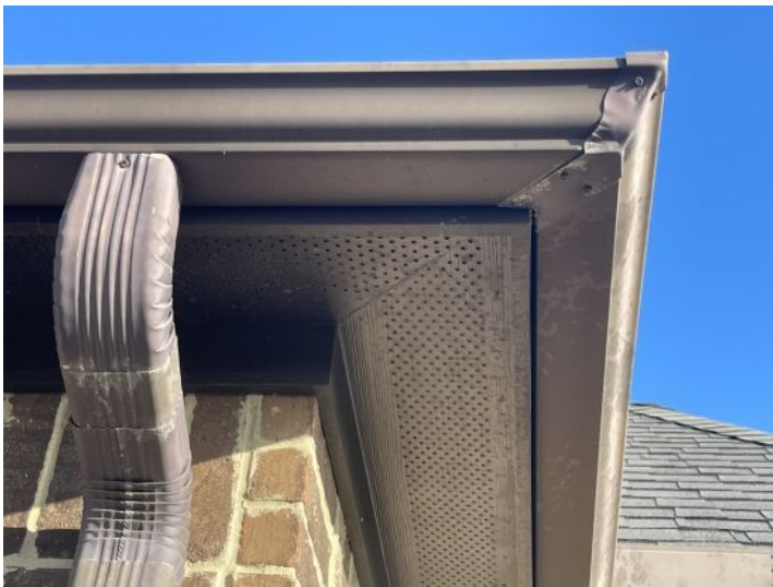
Leaking gutters and downspouts at various locations
