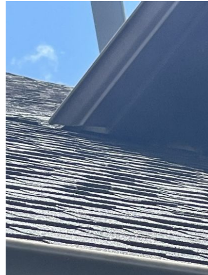
Gutter discharging on roof covering. Recommend evaluation by a gutter contractor and remediation as recommended
