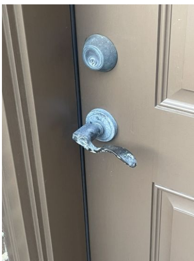
Corroded door hardware - various locations
