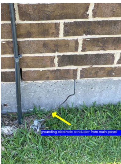
Grounding electrode conductor from main service panel. NOTE - only one electrode present. Recommend upgrade.
