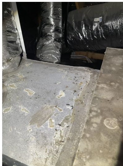
indications of pest activity on HVAC cabinets
