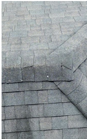
Damaged/split ridge cap shingles - various locations
