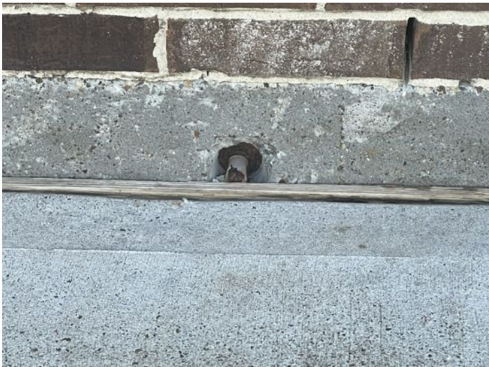
Exposed post-tension cable anchors at various locations
