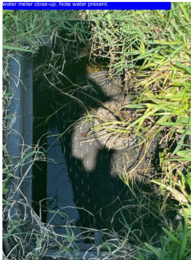
Water meter close up - note loose cover, water standing in meter box due to recent rains
