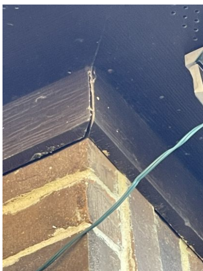
Open joints at frieze boards at various locations. Caulk/seal and monitor
