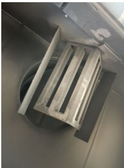
Fireplace flue - recommend installing a damper clamp
