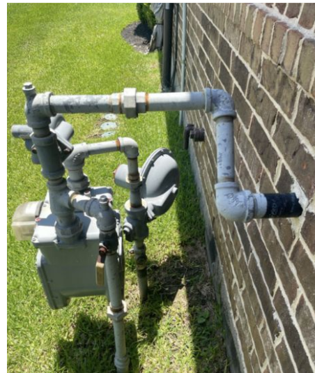
No bonding present at gas meter assembly. Work with a licensed electrician to bond the assembly to the electrical system.
