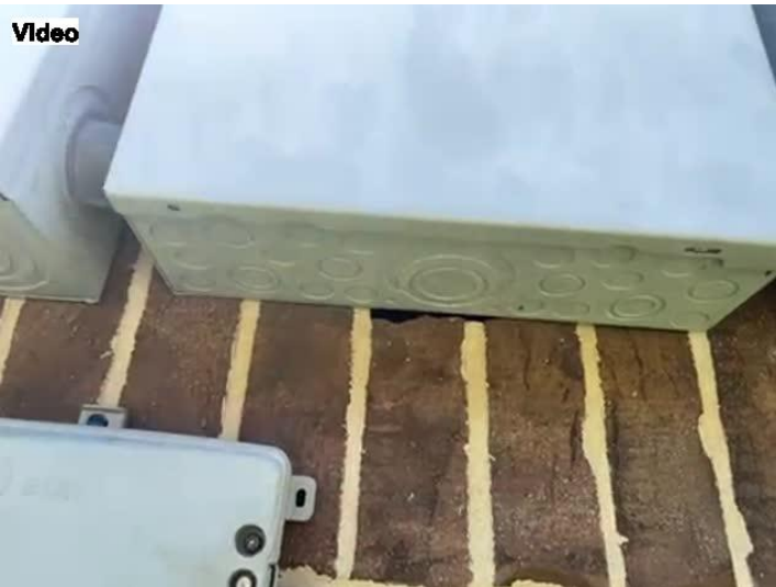
Holes in brick veneer - electrical main and sub panel
