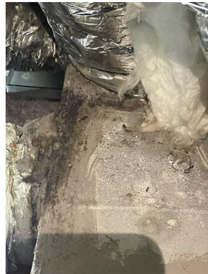
Possible organic growth on HVAC plenum and ducts
