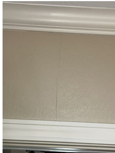
tape joint crack - upstairs hall
