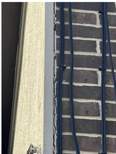
Open caulk joint - stucco to brick interface
