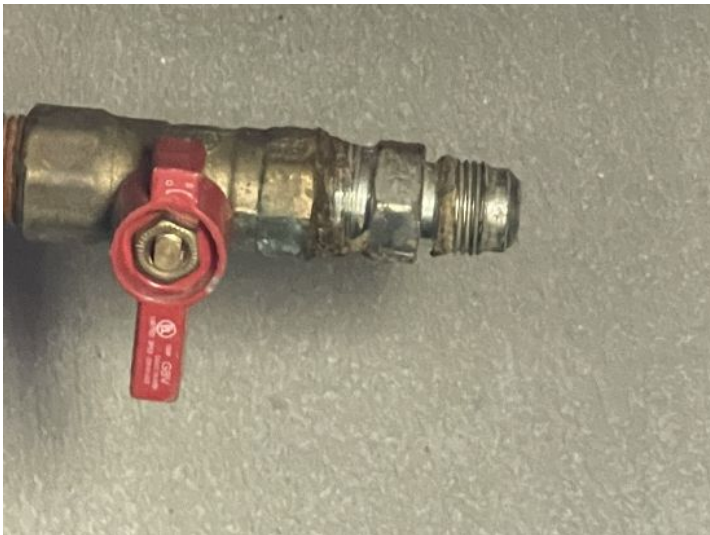
Missing caps at one or more unused gas valves. Cap with approved materials
