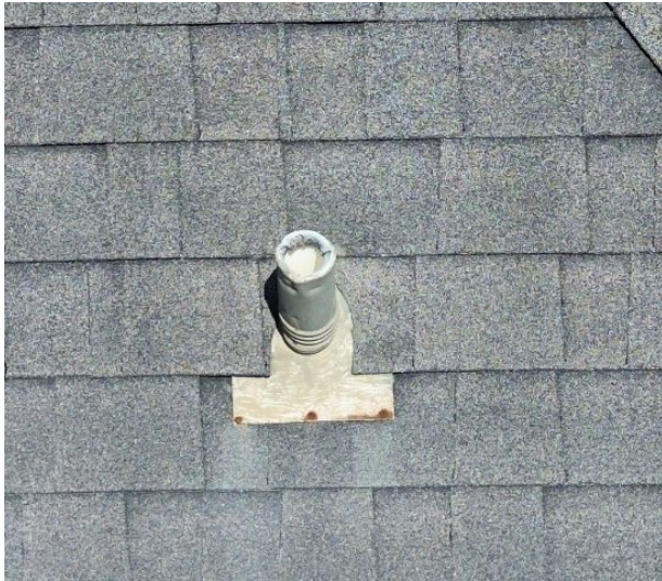
Exposed fasteners at various flashing locations
