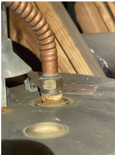
Corroded inlet and outlet pipes at water heaters. Recommend replacing corroded fittings
