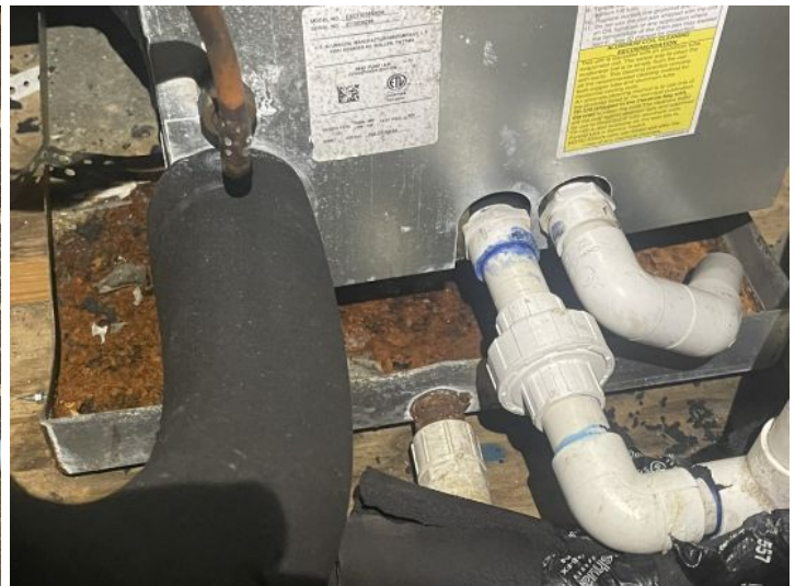
Rust and moisture present in secondary drain pans
