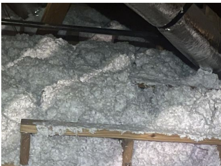
Evidence of pest activity - tunnels and compressed insulation
