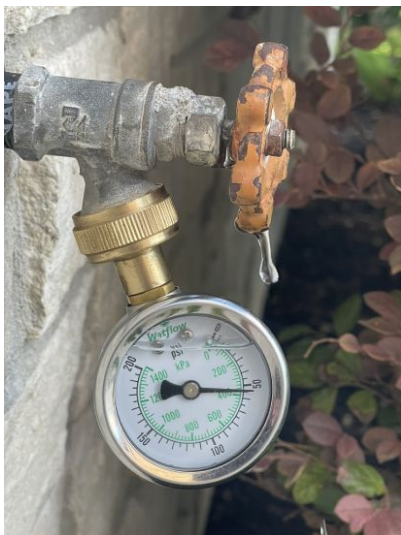
Water pressure of 55 PSI. Note leaking faucet and missing anti-siphon device
