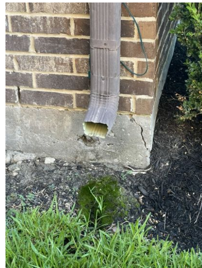
Downspout terminating at foundation. Recommend extending 5 ft from foundation at a splash block
