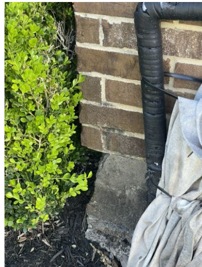
Corner cracks observed at various locations
