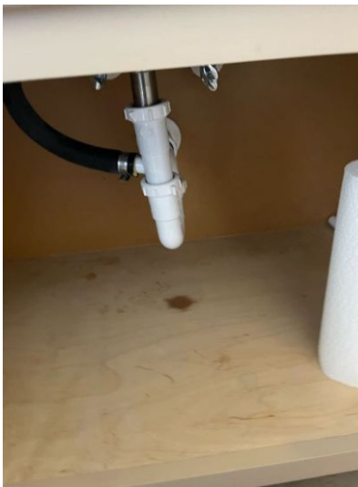
Leak at sink drain - upstairs bath 1
